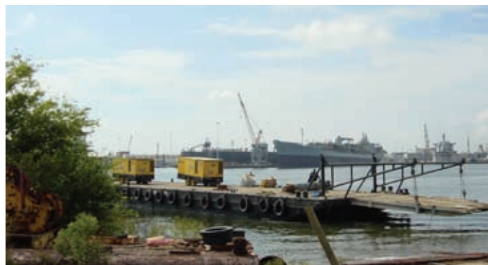
Sunland Construction crews used a barge to transport the Grundoram Taurus pneumatic pipe rammer to the job site for the HDD Assist operation. The crew was attempting a 5,400-ft pullback of 40-in casing when pullback stalled 700 feet short.
