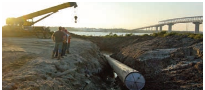
Within ten minute of utilizing the pipe rammer, the immobilized pipe began moving and pullback was successfully completed. Sunland preordered the pipe rammer as an "insurance policy" for this difficult bore.
