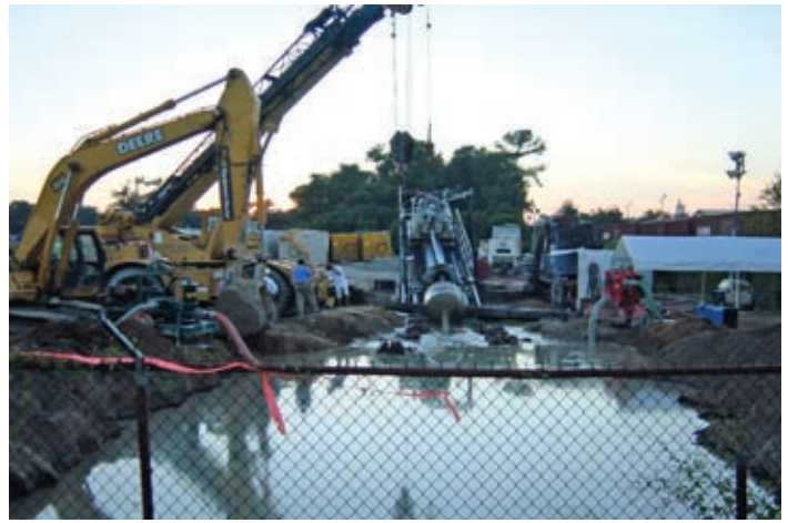
The Sunland Construction crews used a self-manufactured 700,000 lb capacity drill rig for the difficult water main installation project under the Cooper River in South Carolina.
