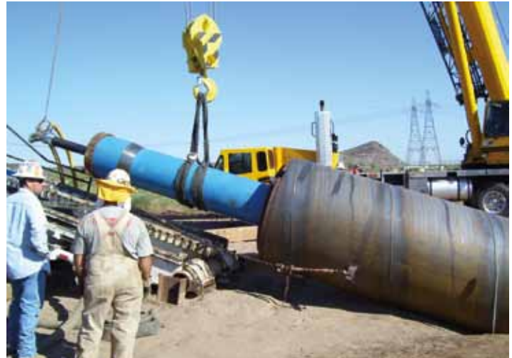
For the 4003-foot Gila River crossing (Phoenix, Ariz.), The Crossing Company installed a 60-inch Conductor Barrel® casing at the beginning of the bore. Crews used a 24-inch Grundoram Taurus to install the casing.
