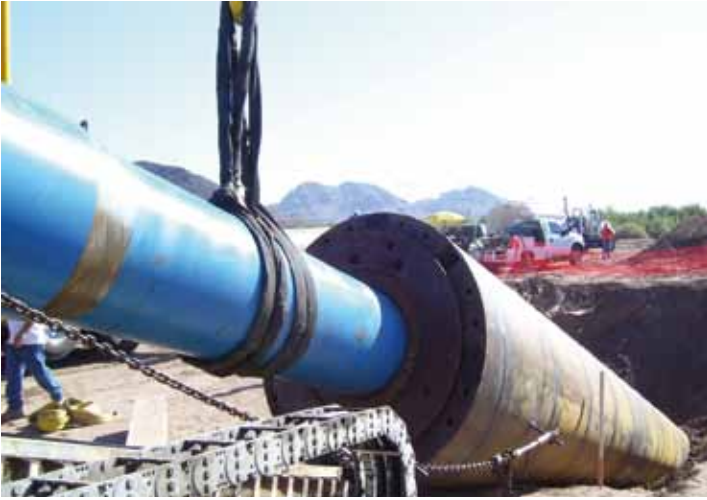
The Taurus ramming tool installed the casing at approximately 30-feet per hour. The total length of casing installed on the Gila River project was 147-feet.
