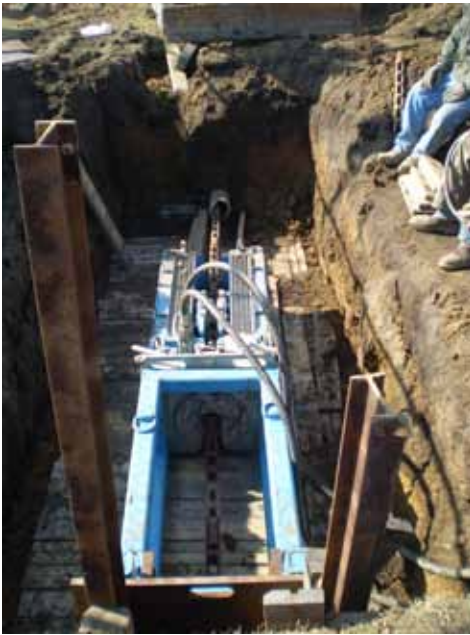
The crews divided the run into two segments, position the bursting unit in the middle. While bursting the first run, crews allowed the Quicklock bursting rods to pass through the machine and rod the second bursting run, a time saving technique.
