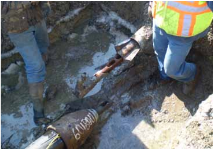
During the static bursting process specially designed bladed rollers are pulled through an existing pipe. As the bladed rollers are pulled through, they split the host pipe and expander attached forces the fragmented pipe into the surrounding soil while simultaneously pulling in the new pipe. Pictured tri-blade cutter, expander and new HDPE.
