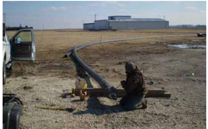
The Herscher storage field expansion project included the replacement and upgrading of a 2,300-foot, 6-inch fiberglass water line to an 8-inch SDR 11 HDPE line through pipe bursting. That particular line distributes water to and from water pump wells and water disposal wells. Pictured staged 8-inch HDPE.
